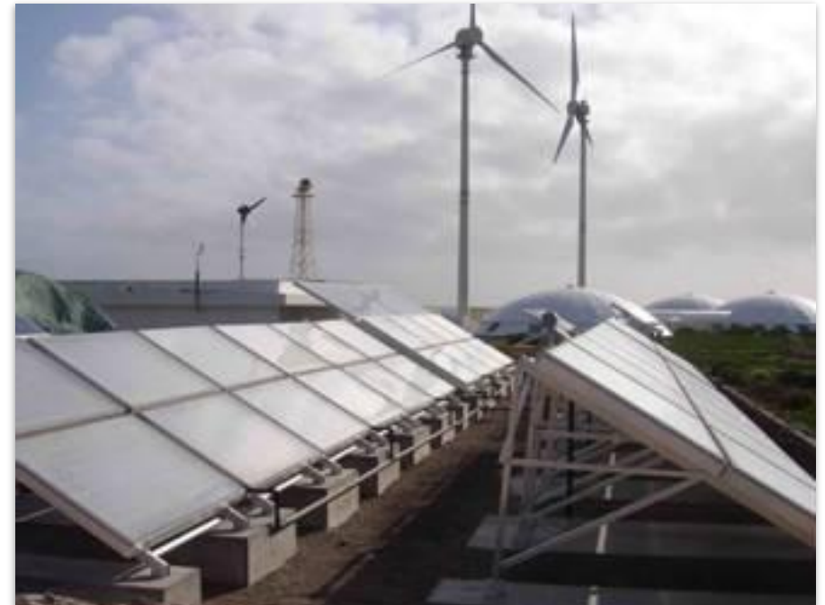
Desalination system for capacities up to 2000 l/day, 90 m 2 , Gran Canaria
